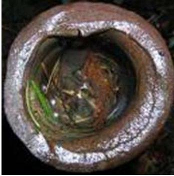
Figure 21. Looking down on an iron pipe corner. The edge is rolled from being hammered.
