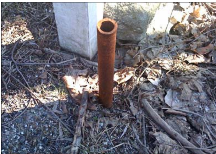
Figure 22. 1 1/4" iron pipe found beside post.
