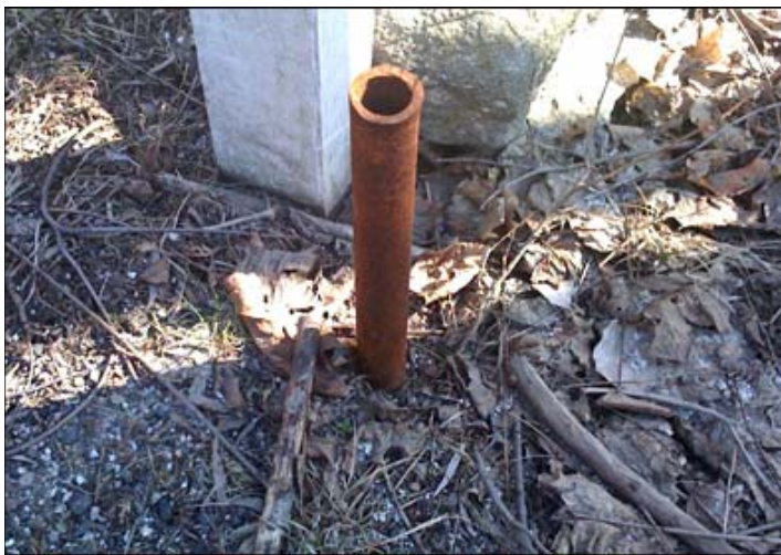
Figure 22. 1 1/4" iron pipe found beside post.
