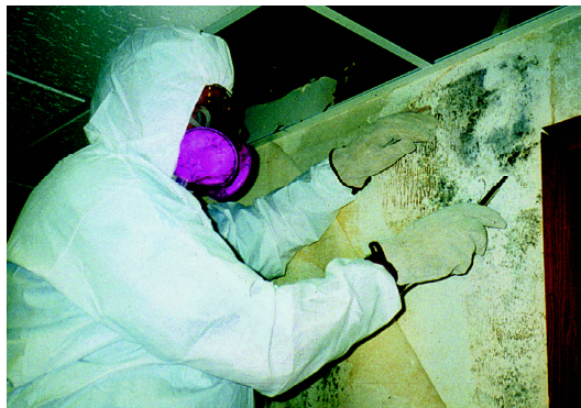
Photo 7: Remediation worker with limited PPE
