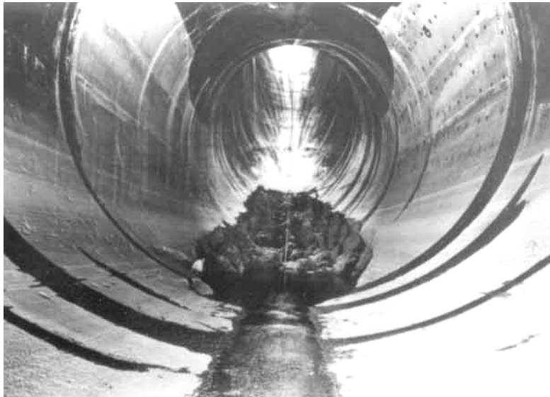
Figure 7 – Axial View of damage in Hoover Dam Spillway (Source: Ref. 3, Fig. 6.5) 11
