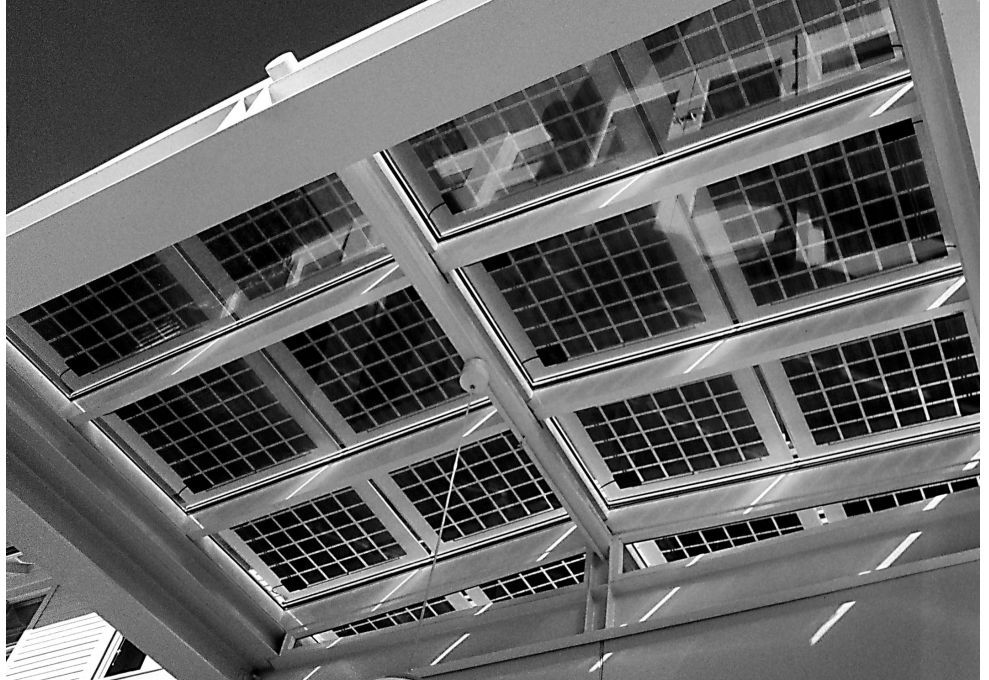
The PV arrays produce electricity and serve as a daylighting design element.
