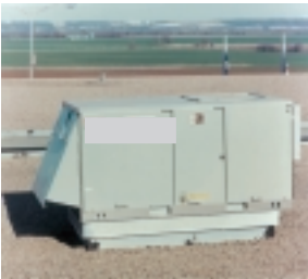
Figure 11: Small rooftop air handling unit.
