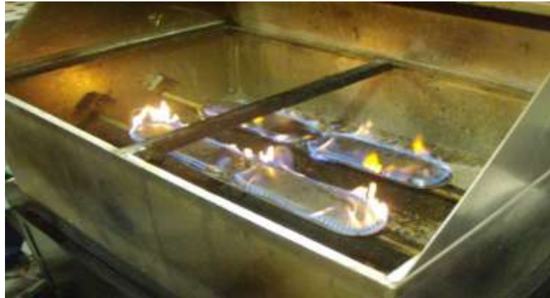
Figure 7 Burners Firing Improperly
