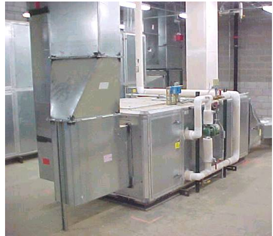
HVAC systems like this can contribute to indoor air quality problems if they are not maintained
