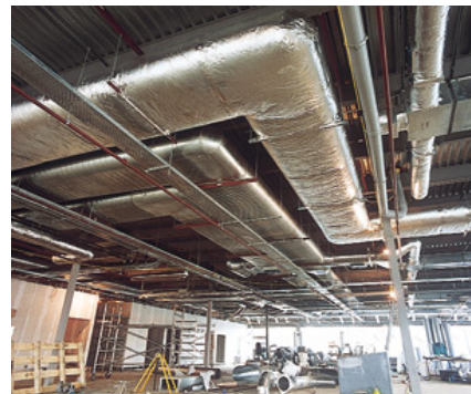
HVAC duct work is another pathway for contamination
