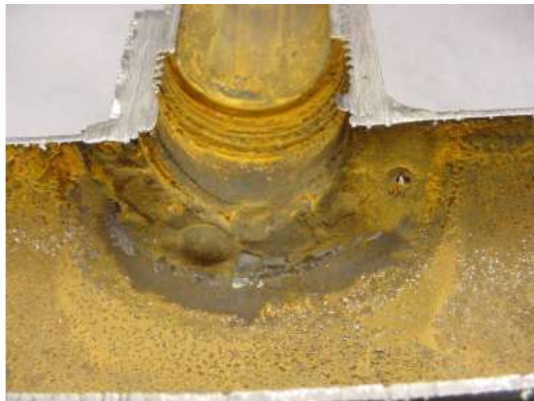
Sectioned head area showing MIC around the weld joint
