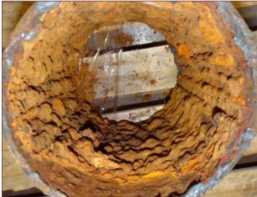
Photograph showing tubercle formation in a water line
