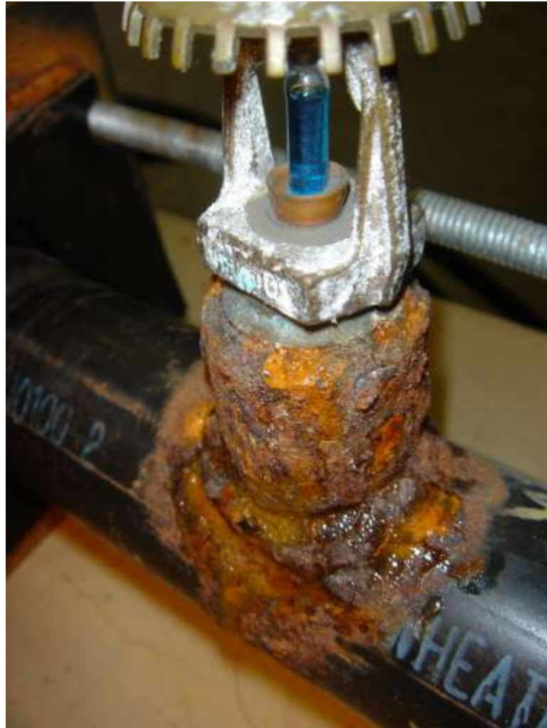
Photograph showing corrosion on sprinkler pipe
