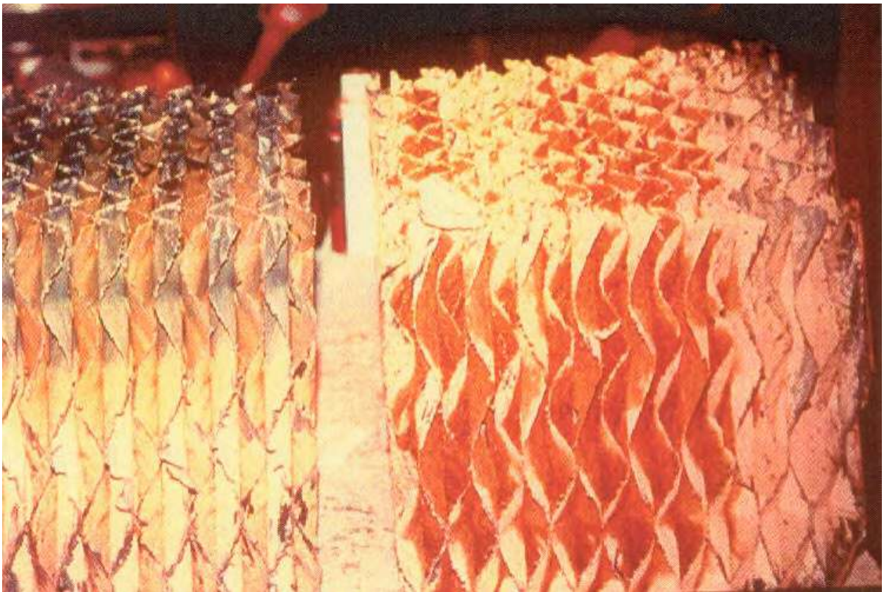
Figure 14 Heavily Fouled Cooling Tower Film Fill
