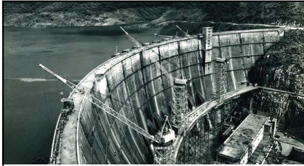
Above: about two-hundred and sixty miles northwest of Bangkok, Thailand, a crew of 4K men built a huge new dam and power plant known as the “Yanhee Multipurpose Project.” The $100 million undertaking included two Otis passenger elevators for maintenance purposes. When the dam was completed in 1964, it was the largest of its kind in Southeast Asia. 979
