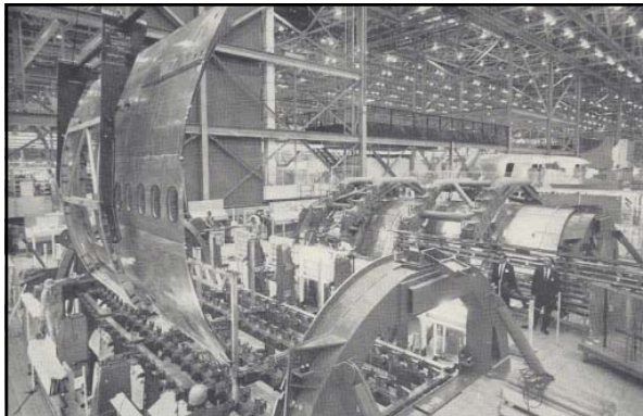
Above: caption: "Fuselage panel made by Northrop Corp. is eased into section 44 build-up fixture using crane. This is typical of the way all fuselage sections are assembled. Large size of 747 components has required greater use of overhead cranes than anticipated." 441
