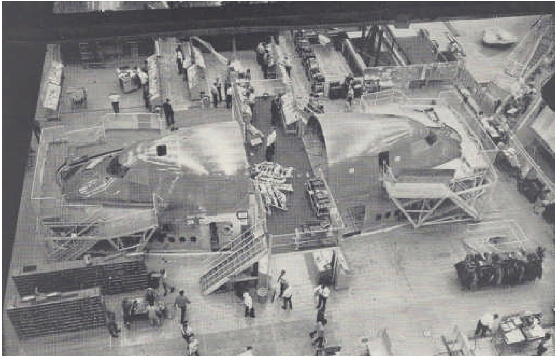
Above: caption: “Cab sections made in Boeing’s Wichita plant have bulk of wiring, tubing, insulation and the like installed prior to mating with the main fuselage. Work platform level is at the same height as the main floor of the cab.”
