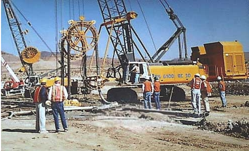
Figure 2: Example of the type of heavy track-mounted equipment that needs special handling to get on site and assemble for use. This equipment was operated to dig and install a cut-off wall in the foundation of a major dam.
