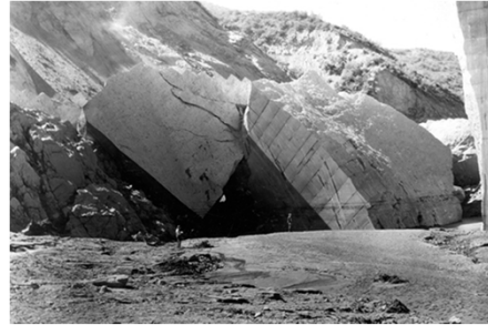
St. Francis Dam, Concrete Debris Blocks (Attribution: U.S. Geological Survey Photographic Library)
