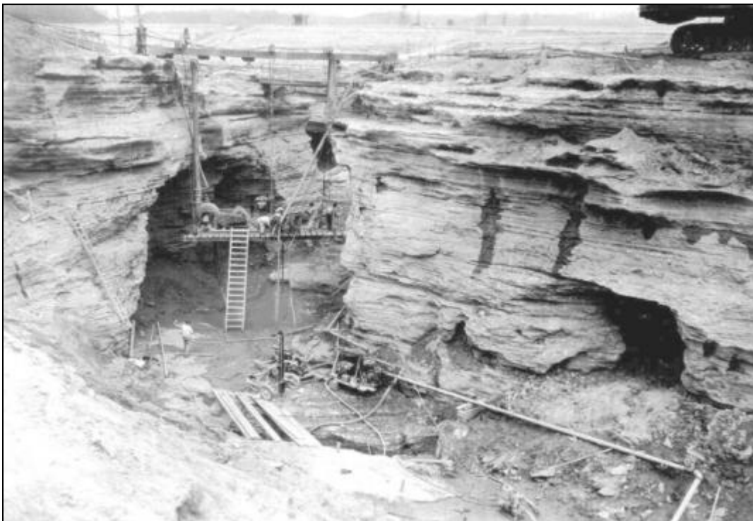
Figure 17-24. Foundation treatment of a network of caves and dissolution channels at Wolf Creek Dam as part of original construction (Nashville District).
