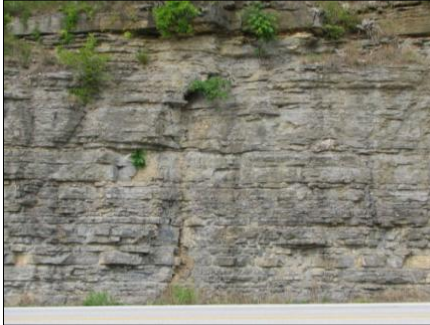
Figure 17-17. Large expanse of minimally dissolved rock at Center Hill Dam (Nashville District).
