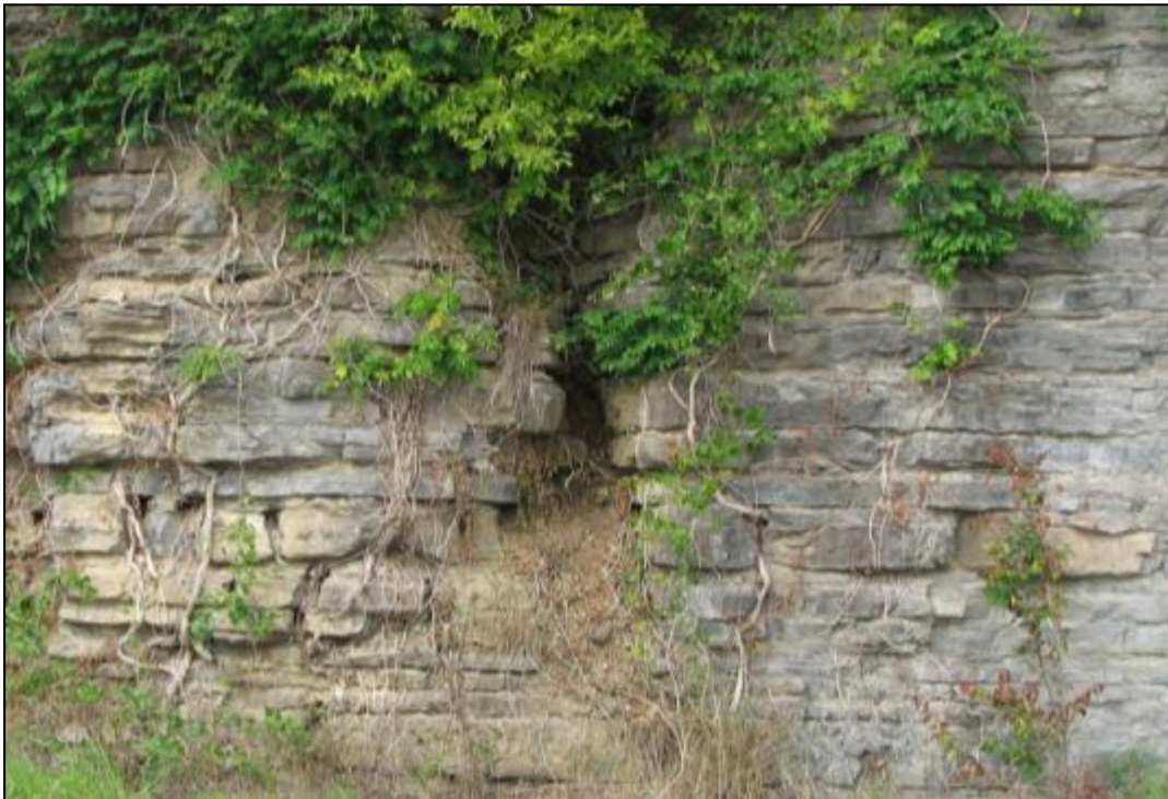
Figure 17-12. Near-surface vertical feature at Center Hill Dam (Nashville District).
