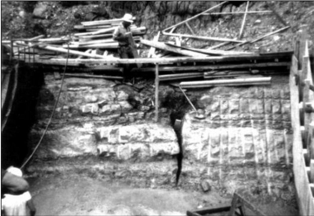
Figure 17-23. Triangular dissolution feature in the excavation sidewall of Mississinewa Dam, treated at the time of original construction (Louisville District).
