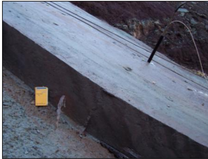
Figure 7-7. Leaky grout cap caused by improper concrete consolidation.
