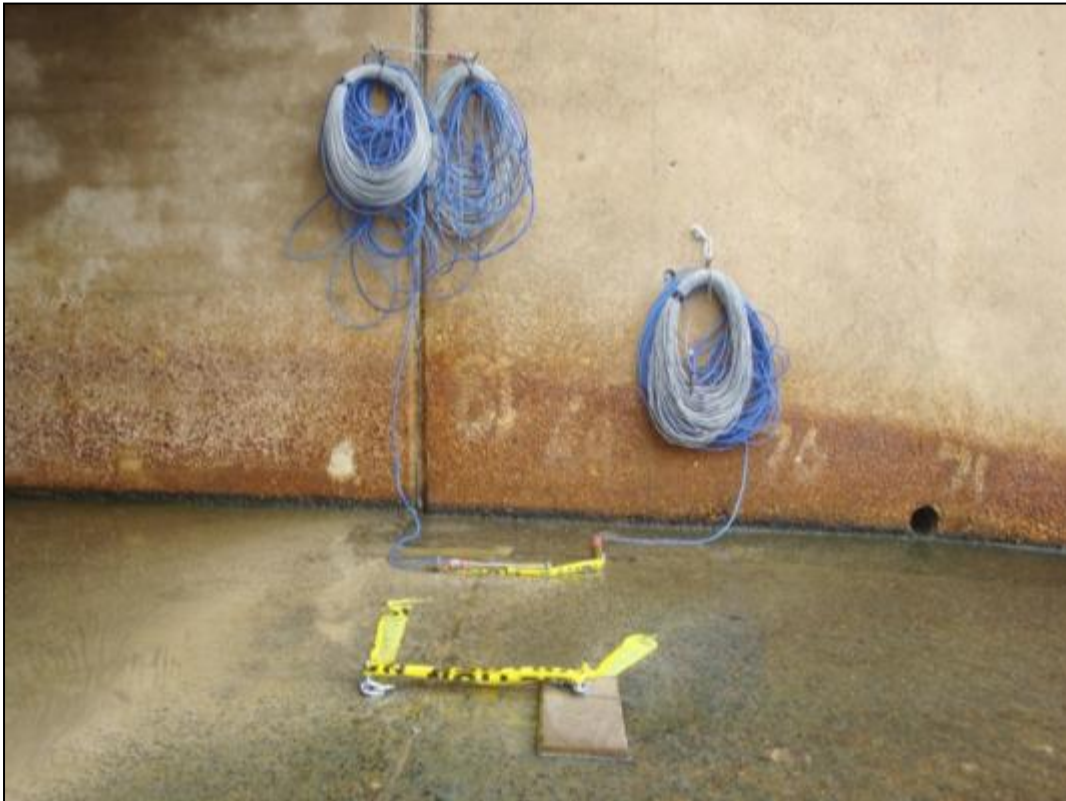
Figure 25-6. Crack displacement devices installed at the spillway wall and parabolic slab at Barker Dam west of Houston, TX (Galveston District). The instruments were monitored in real time during grouting to ensure that there was no movement or displacement of the walls and slab.
