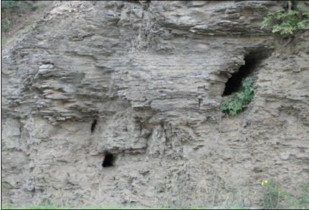
Figure 17-15. Isolated dissolution features along the structure at Wolf Creek Dam (Nashville District).
