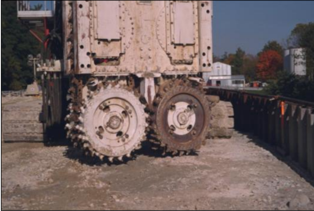
Figure 19-3. Hydromill cutter wheels for limestone excavation at the Mississinewa Dam cutoff wall (Louisville District).
