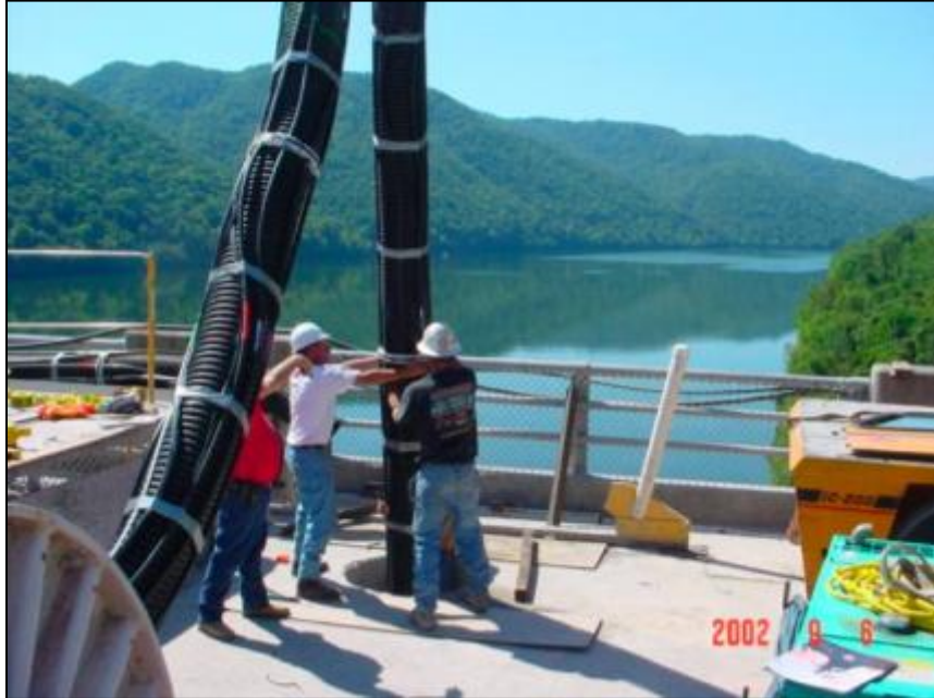
Figure 23-7. Corrugated duct being inserted into the prepared anchor hole at Bluestone Dam, WV (Huntington District). The numerous external tremie tubes are clearly visible.
