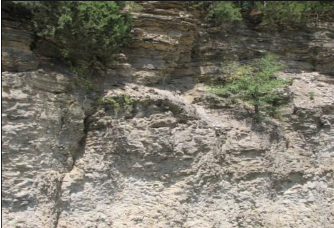
Figure 17-16. Isolated near-vertical dissolution along the structure at Wolf Creek Dam (Nashville District).
