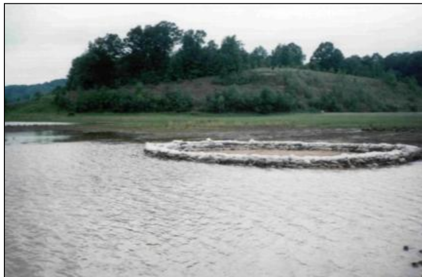
Figure 17-6. Sandbagged dropout sinkhole that developed in an emergency spillway approach channel during a flood at Patoka Dam (Louisville District).
