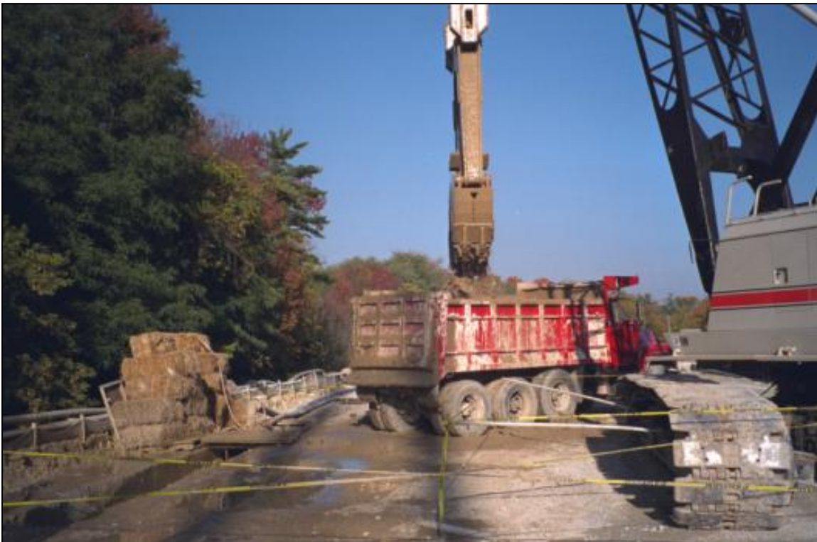
Figure 19-2. Cable-operated clamshell for overburden excavation at the Mississinewa Dam cutoff wall (Louisville District).
