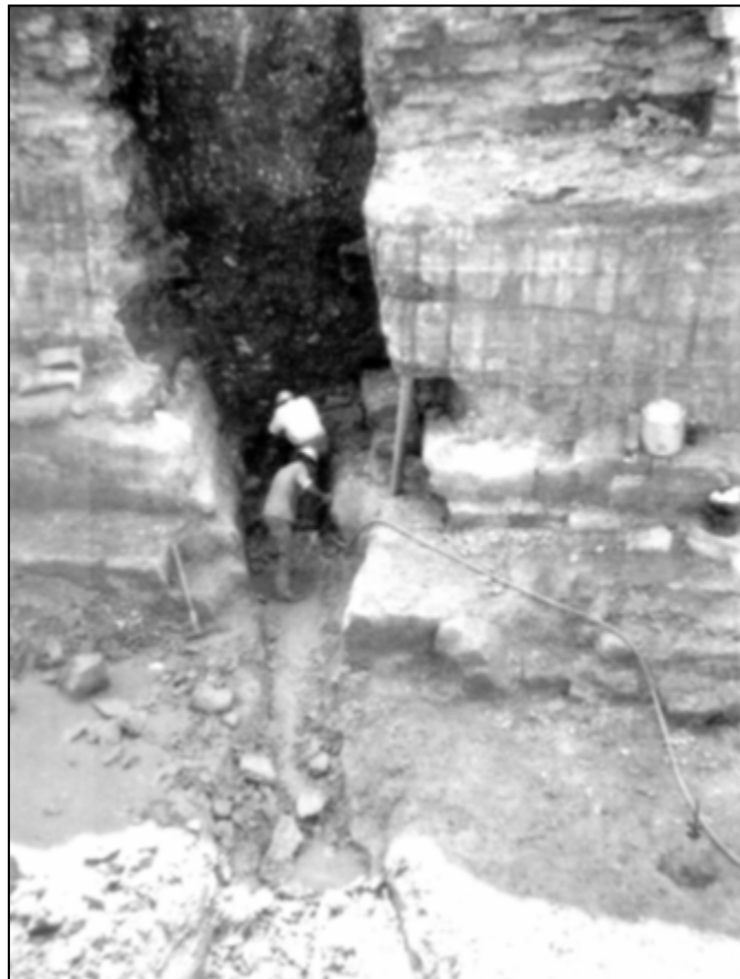
Figure 17-22. Triangular dissolution feature in the foundation of Mississinewa Dam, treated at the time of original construction (Louisville District).
