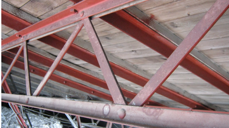
Example of Locally Fabricated Riveted Joist from the Chester County Courthouse, PA
