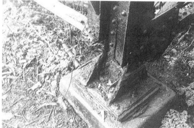
Wrought Iron Deterioration
