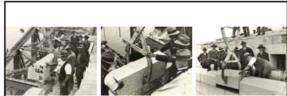
Setting of the last stone, February 1932 Stonemason foreman Jock Mackay lays the last block of granite on the NW Pylon. Looking on are JJC Bradfield, Lawrence Ennis, RJ Butler and James Muir. On February 6, 1932 (a week earlier) rigger foreman James Campbell (while dismantling a derrick crane) was knocked off the Pylon when a gust of wind caught the crane. The ceremony was held in the spot where he fell to his death to honor his memory and his faithful service. 350
