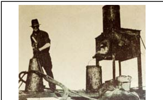
Heating a rivet to “white hot” (in an oven) and passing to boilermaker (inside chord/s) pneumatically via flexible metal tubing
