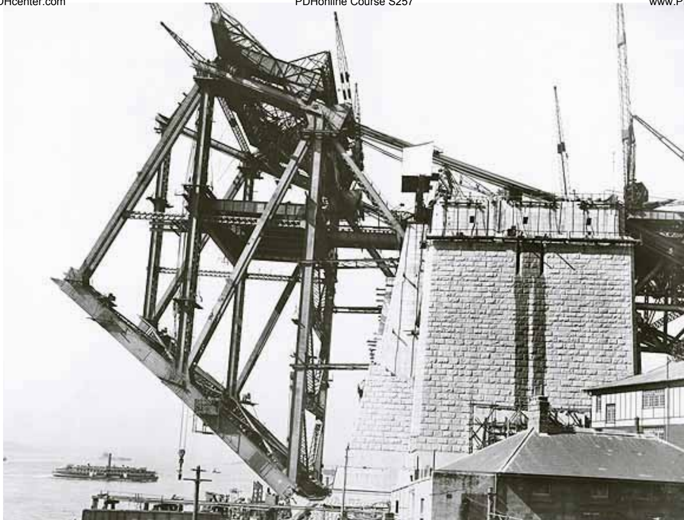
Creeper crane atop first (arch) panel Ramp removed and wire cables in-place
