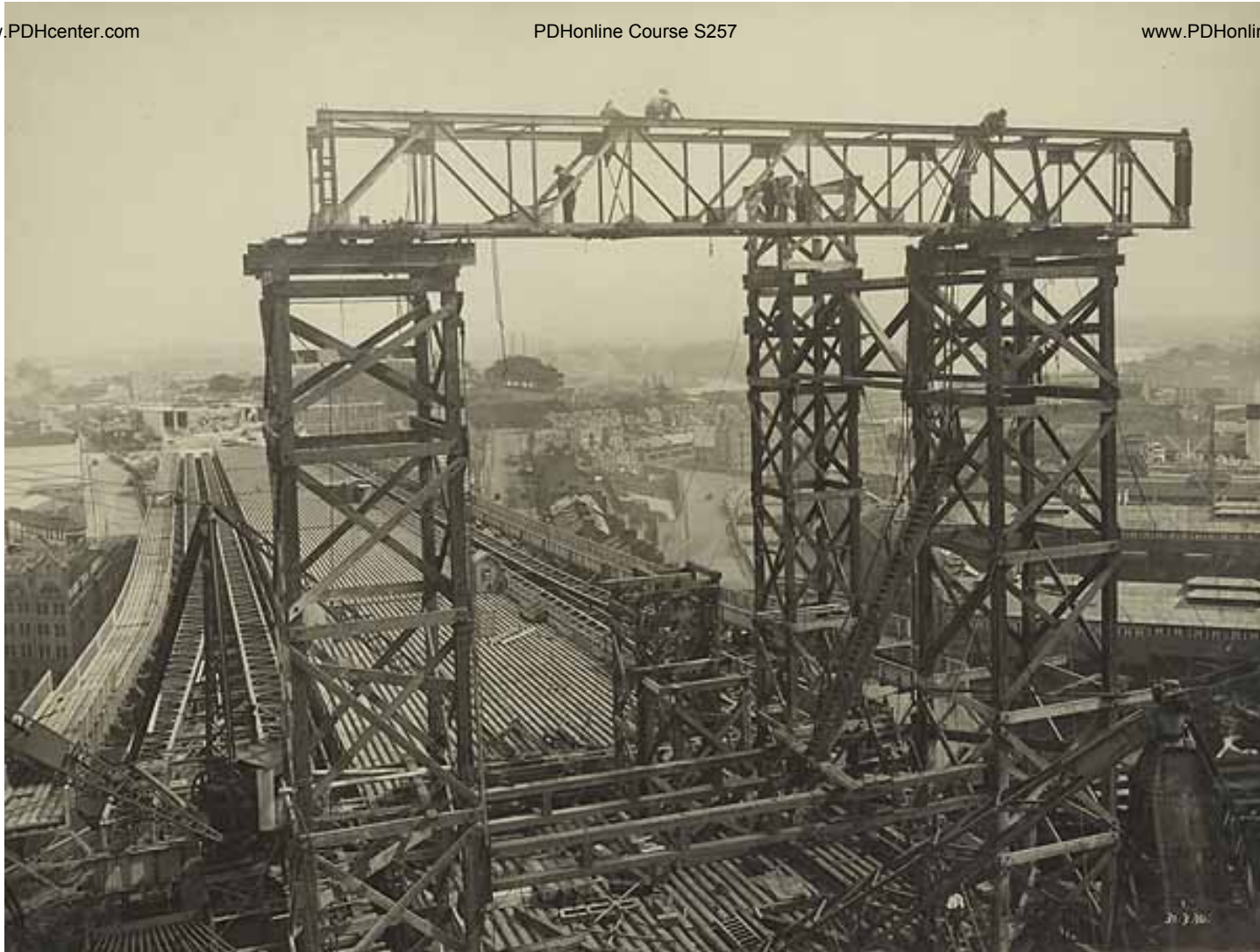
Temporary framework (between Pylon towers) for support of two hoisting cranes (set atop) 346
