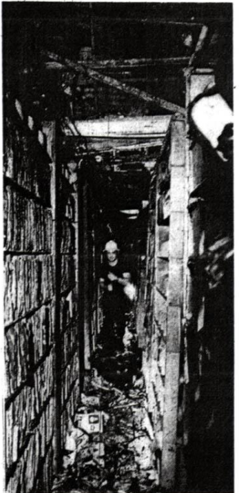
The New York Times/Terrace Dubois A Port Authority workman stringing temporary lighting wires inside storage and telephone switching room of R. J. Saunders, Inc., on eleventh floor of north tower of World Trade Center. Fire may have started here.
