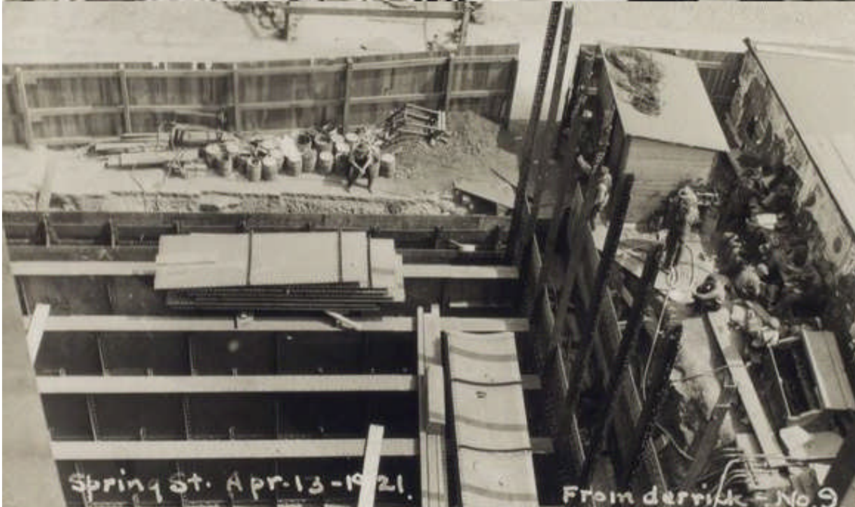
Bottom: caption: “Roof girders and sided angles, roof plates on blocking. Spring Street, April 13, 1921”
