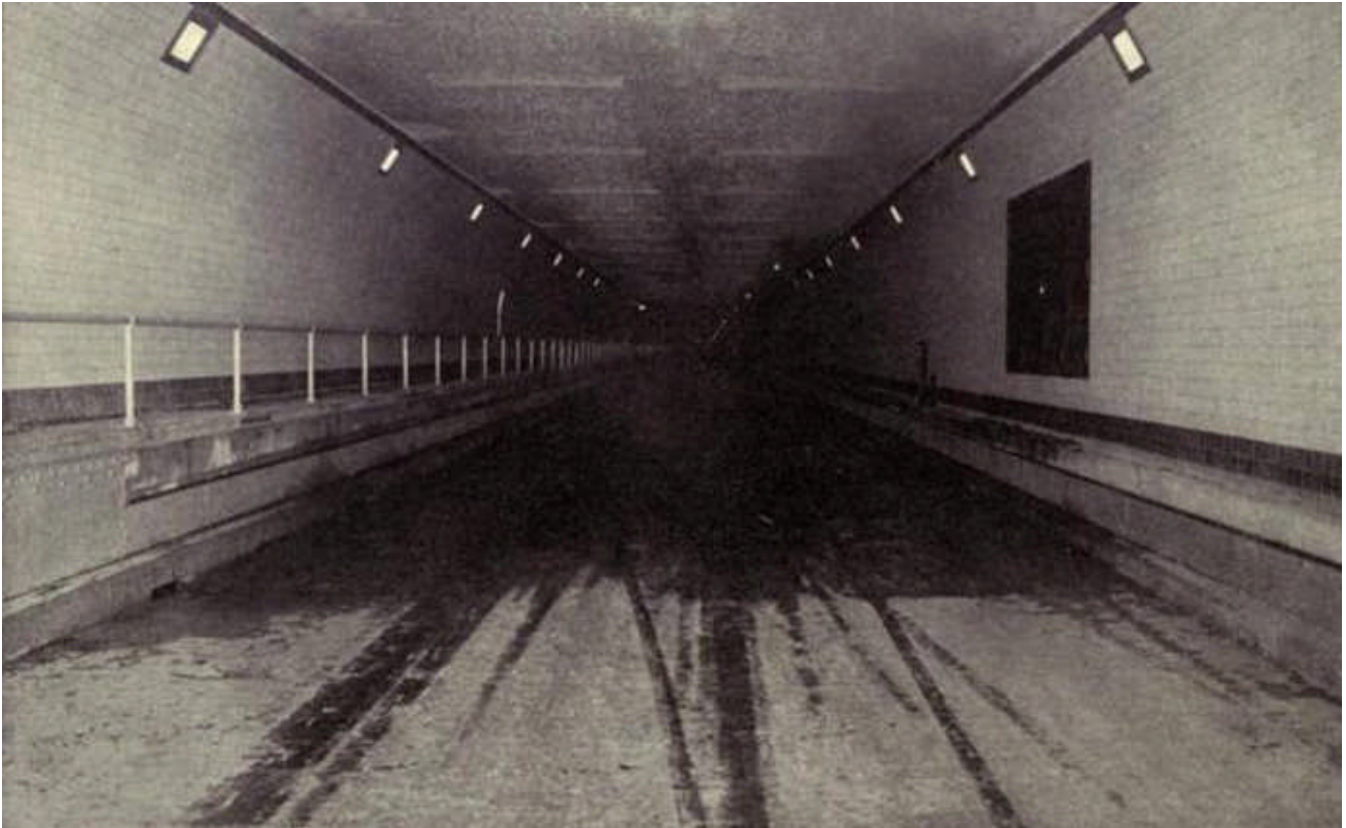
Above: caption: “Condensation in North Tunnel. View showing dry conditions of roadway east of air duct bulkhead where fans were in operation, and wet conditions on roadway west of air duct bulkhead where fans were not in operation.”
