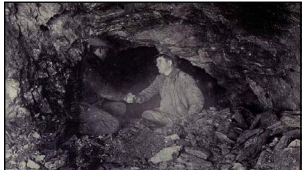
Above: caption: "Holing Through! Tunnel superintendent Harry Redwood, of New York side, shaking hands with Norman Redwood, of New Jersey side, North Tunnel" 574
