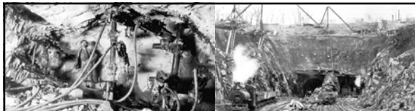
The tunneling crews worked from both ends of each tunnel, drilling into the hard rock with Rand "slugger" compressed-air drills. Then, dynamite was placed to break up the rock. Typically, tunnel headings were first drilled and blasted horizontally to form the upper section of the tunnel and then drilled and blasted vertically behind this heading on two "bench" levels to excavate the full tunnel section. Steam shovels loaded the excavated rock into 3-foot gauge muck trains, which were pulled out to tunnel portals by 12-ton "Vulcan" steam locomotives. The hard traprock was stored and later crushed for use as concrete aggregate and track ballast. Drilling through Bergen Hill proved tedious and costly. Progress was only from 2 to 7-feet per day and the tunnels were not finished until the end of 1908 (they were begun in early 1905).
