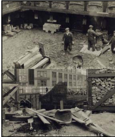
Top: caption: "Working chamber, Cutting edge, Blocking, Canal Street, May 6, 1921" Bottom: caption: "West side, inner and outer skin plates. Canal Street, May 6, 1921"
