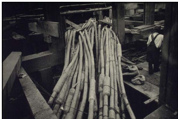
Above: caption: "N.Y. Telephone Co. cables at Canal & Hudson Streets, New York. 12/2/24." 497
