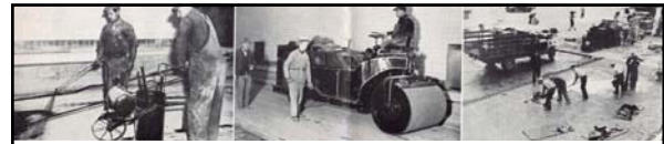
Above Left-to-Right: caption: "Pressure spraying base with bituminous prime coat before depositing mastic cushion material / Rolling brick on 1-inch surfaced boards with less than ten per cent renewal on entire job / Filler application and surface removal at Weehawken (N.J.) plaza, 180 by 286 feet"
