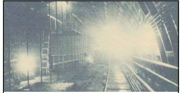
Above: caption: "A great roadway for the motorist of 1938 begins to assume form in the mud and rock of the Hudson River bed: a view in the new Midtown Hudson Tunnel, which has advanced about 200 feet from the New Jersey side of the river and about 600 feet from the Weehawken Terminal Point. The daily movement toward the middle of the river is about twenty-five feet, and great rings of steel are set in place at regular distances for the frame of the tunnel." 806
