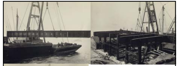
Above L&R: caption: "River Ventilation Building, New York. Erection of steel girders. 3/12/26." Left: caption: "River Ventilation Building, New York. Erection of steel to third floor level. 4/20/26." 550
