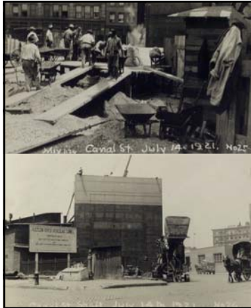
Top: caption: "Concreting, mixing plant. Canal Street, July 14, 1921" Bottom: caption: "Painting. Canal Street Shaft, July 14, 1921"
