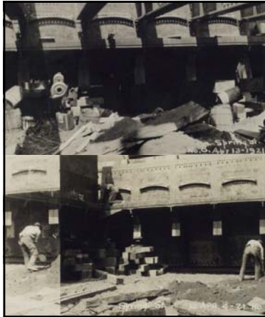
Top: caption: "Working chamber, roof girders bolted. Spring Street, April 13, 1921" Bottom: caption: "Working Chamber, blocking up for bolting, April 13, 1921"
