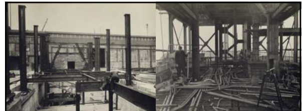
Top Left: caption: "River Ventilation Building. Steel columns for Pier Deck and mezzanine floors, N.Y., New York. 5/28/26." Top Right: caption: "Progress of placing electrical conduits in River Ventilation Building, New York. 6/5/26." Left: caption: "River Ventilation Building, Pierhead Line between Piers 34 and 35, North River, New York. 11/17/26." 552
