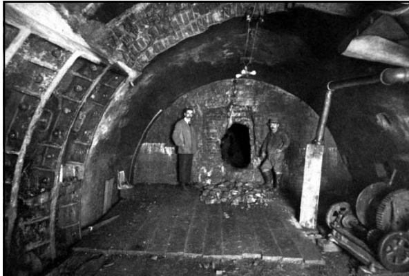
Above: caption: "The south tunnel holed through, breaking into the brick bulkhead at the Morton Street shaft. The newly completed tunnel is in the foreground." 157
