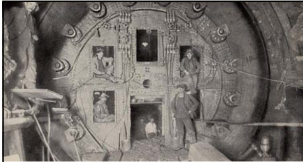
Above: caption: "View of shield used in tunnel construction." One of the greatest improvements in connection with the shield method of tunneling was the use of cast-iron lining by Peter Barlow in 1869 (used in the Thames Tunnel). Lord Cochrane first suggested the use of compressed-air and in 1830, he took out a patent for air-locks and other appliances to be used in tunneling. The next great step in tunneling technology was made in 1887 when an improved shield was invented by J.H. Greathead.
