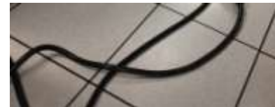
Feeder and branch-circuit cables used for temporary wiring are not permitted on floors or on the ground.
