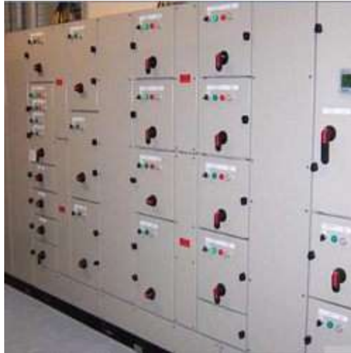
A Typical Motor Control Center
