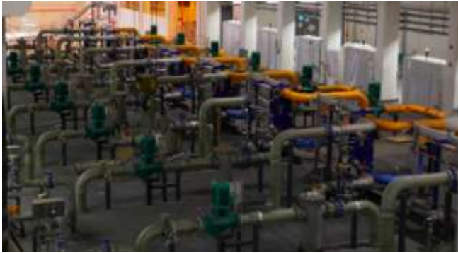
Figure 7: Inside the data center cooling plant; rows of pumps flank their associated heat exchanger.
