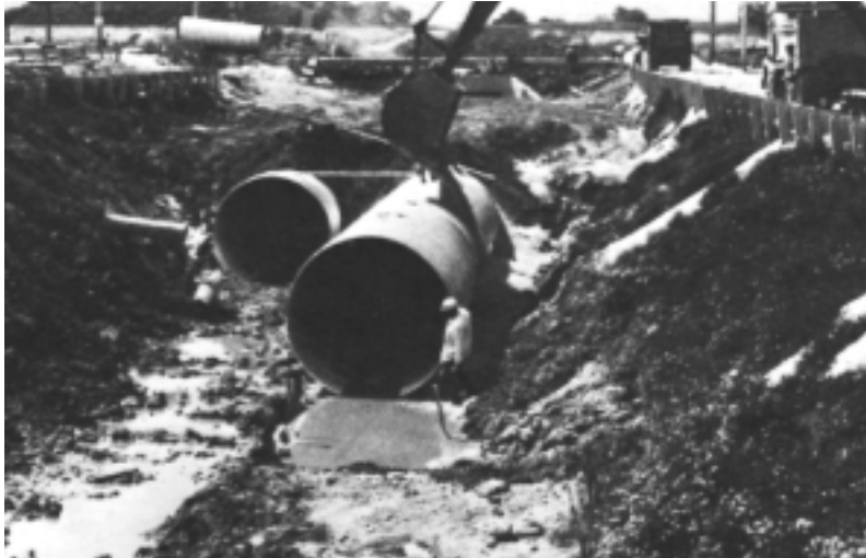
Plain galvanized CSP satisfied service life requirements for storm drains in this environment.
