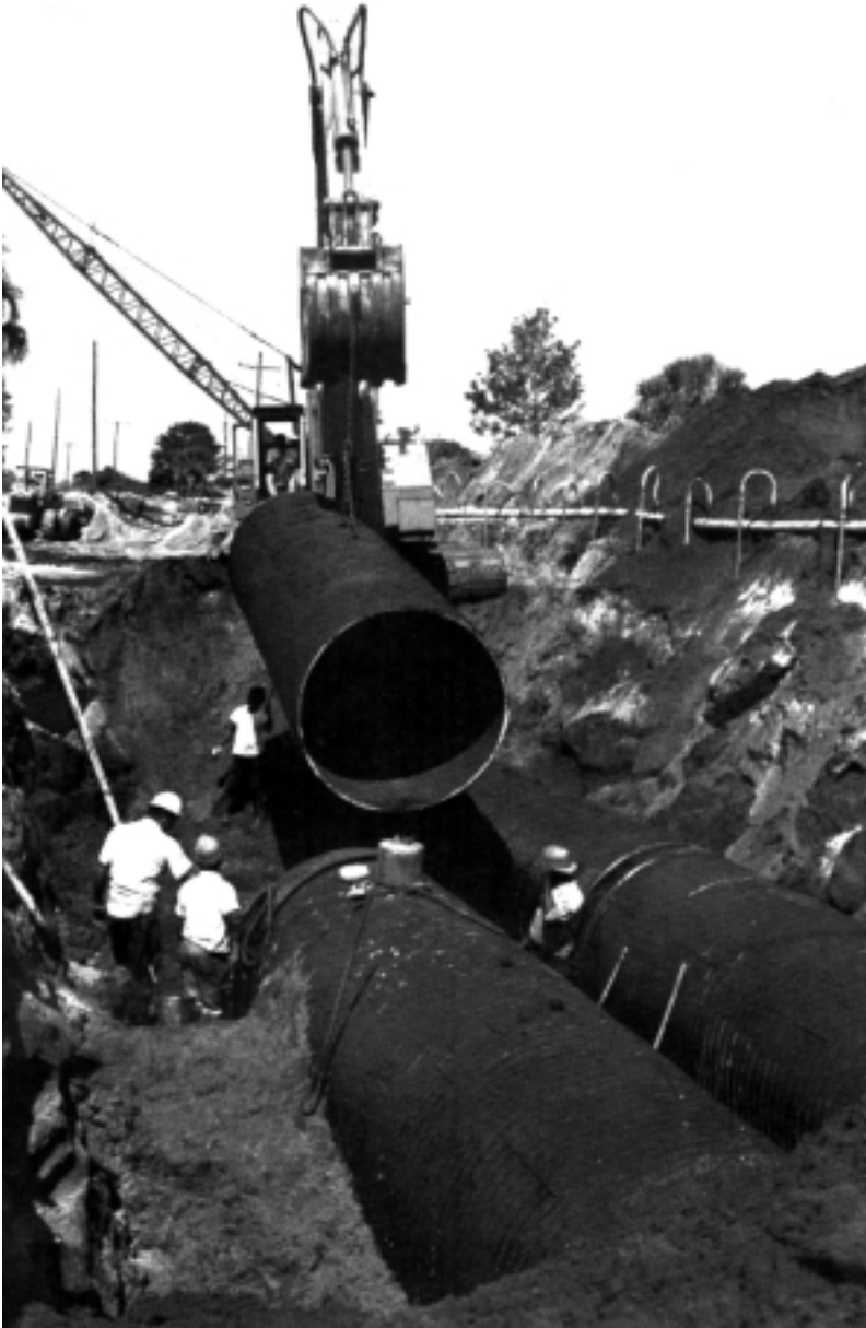
Well points and wide trenches were necessary to install full-bituminous coated and full-paved CSP in this unstable ground.
